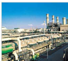
Refinery Plant, Oil-Gas Plant,
